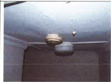
Sagging and damaged ceiling
