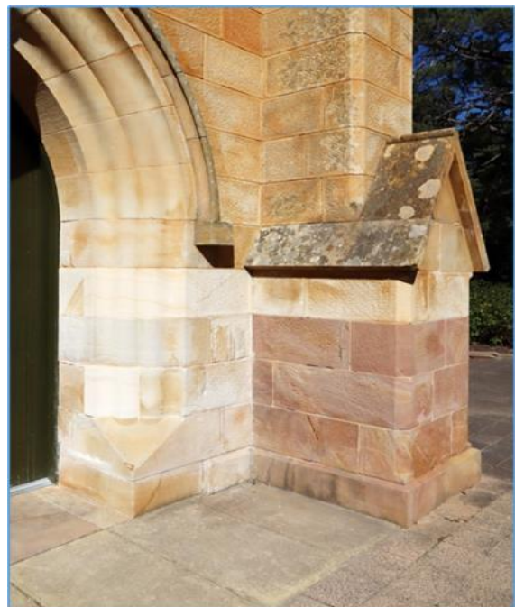
The finished job at the entry arch: after use of a poultice, new slip stones were inserted accompanied by the use of softer, lime mortar.
